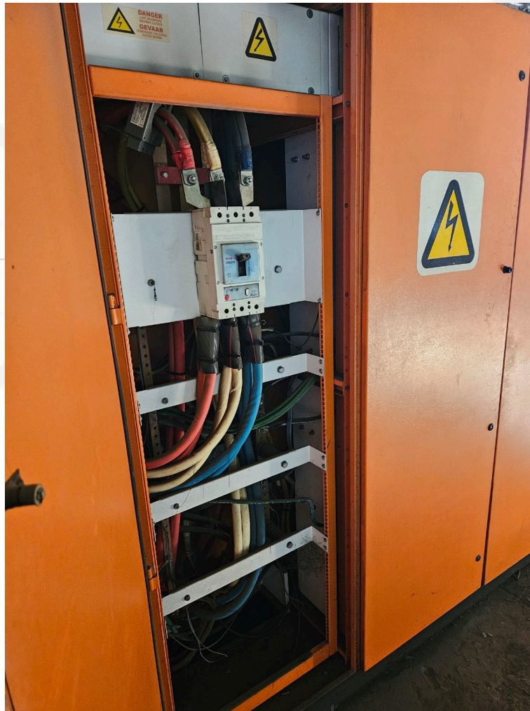
Factory distribution box
