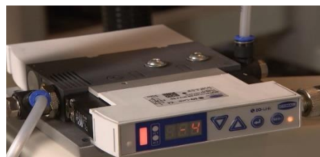
Figure 1: Compressed air leaks
